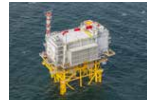
Offshore Wind Substations
