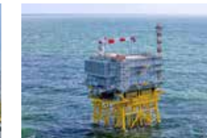
Offshore Wind Substations
