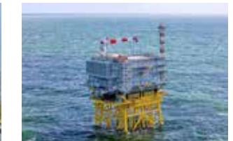
Offshore Wind Substations
